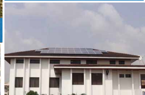
Ghana 10KW PV System
