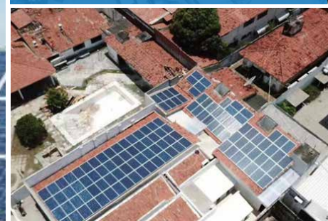
Brazil Roof PV Project
